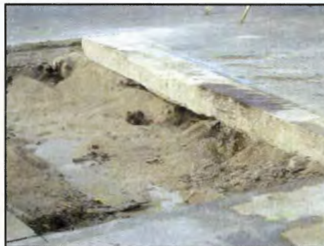
Figure 45. Backfill material caving in on trench edges.
