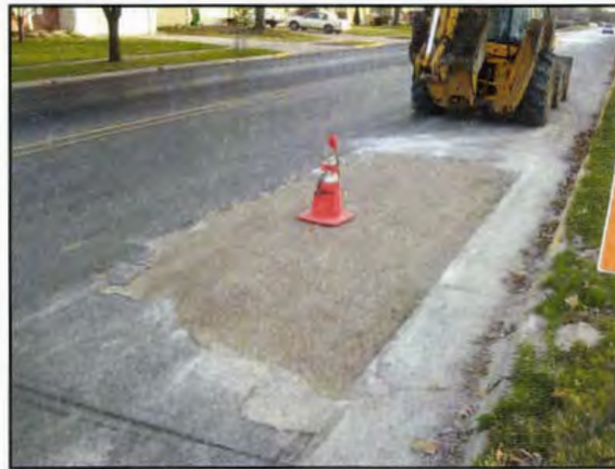
Figure 30. Utility cut left open for two weeks.
