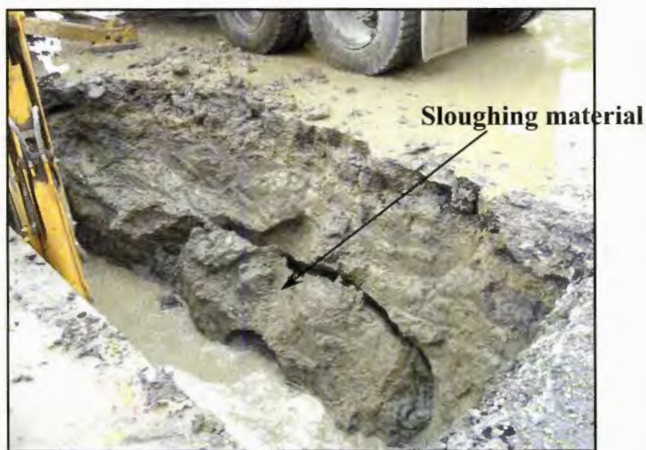
Figure 24. Material sloughing off in Ames site.
