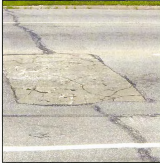
Figure 5. Temporary cold patch in Cedar Rapids.
