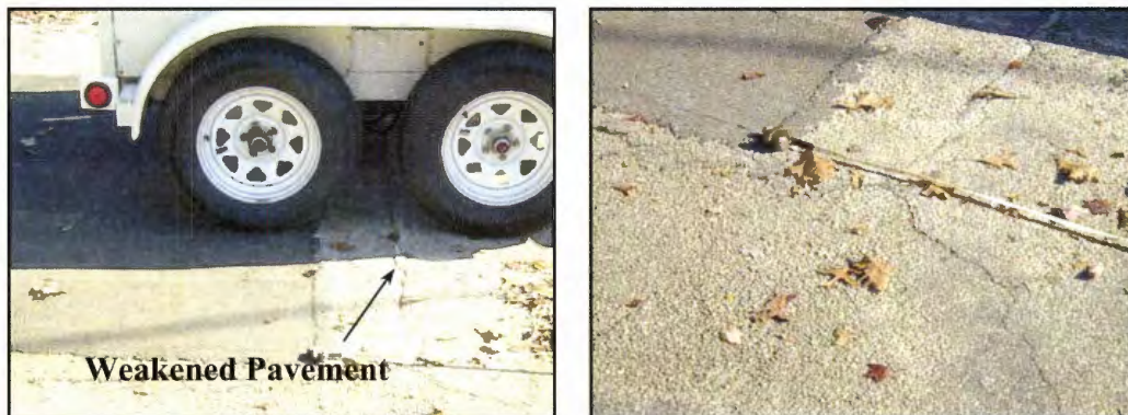
Figure 63. Cedar Rapids pavement distress.
