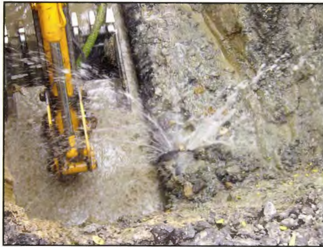
Figure 25. Ames water main break.
