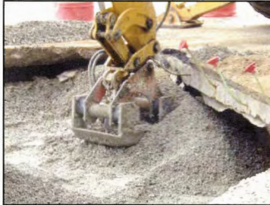
Figure 44. Large cavities forming beneath pavement.
