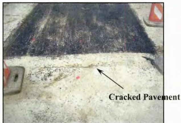
Figure 42. Visible pavement damage on utility edge.
